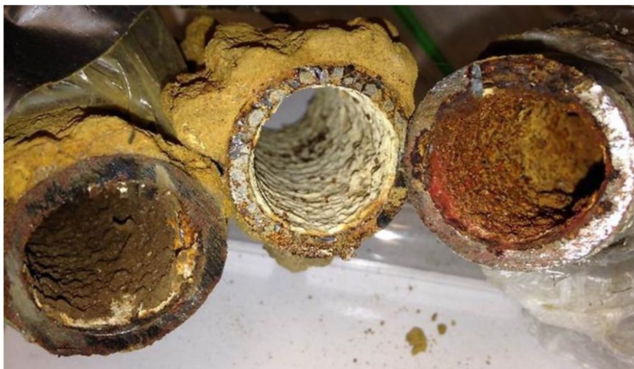
"Flint drinking water pipes." VCU Capital News Service. May 27, 2017. CC BY-NC 2.0)
